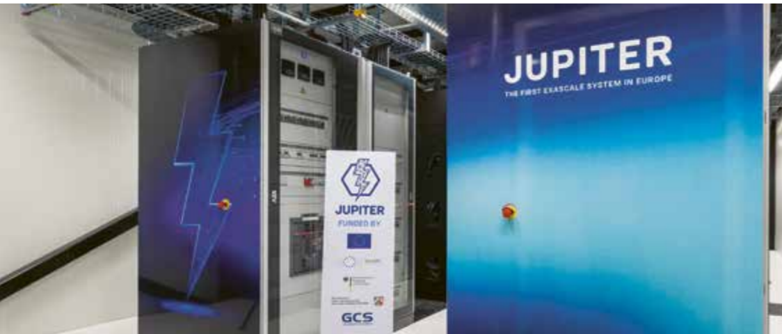
Modular Supercomputer JUPITER at the Jülich Supercomputing Centre.
