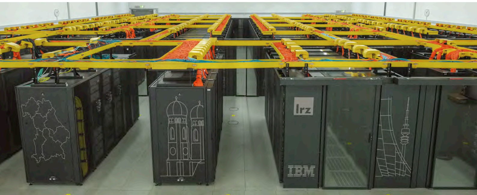
Picture of the Petascale system SuperMUC at the Leibniz Supercomputing Centre.
